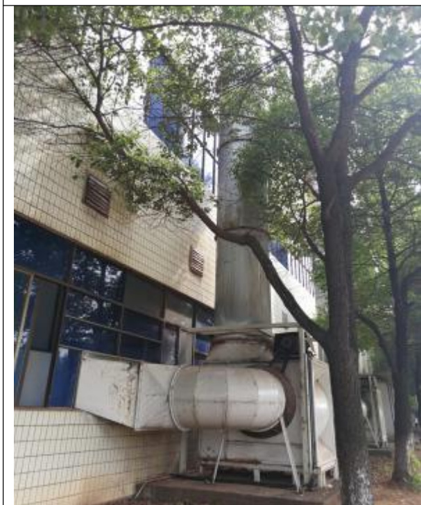
面漆房废气⑤ 排气筒
